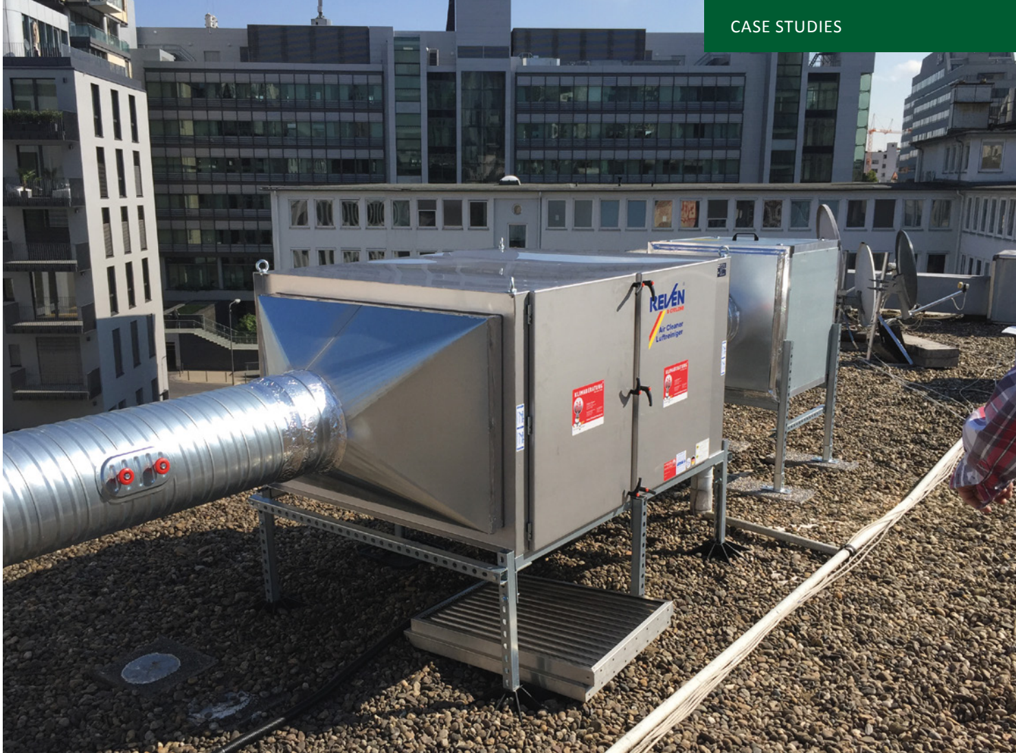
Fully installed duct separator and fan in the exhaust air section of Thai restaurant Aroydee on the roof.
