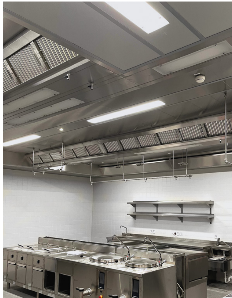
Kitchen ventilation ceiling with RSC and fire-extinguishing system
