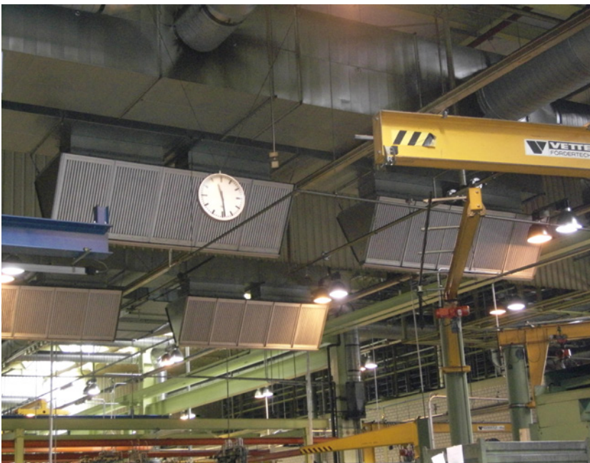
Hall ventilation with fume capture modules from the X-CYCLONE® E2S series
