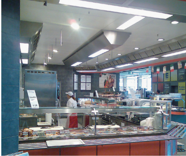
Ventilation ceiling for a canteen serving area
