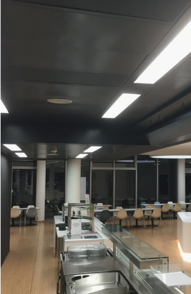
Black ventilation ceiling in a canteen
