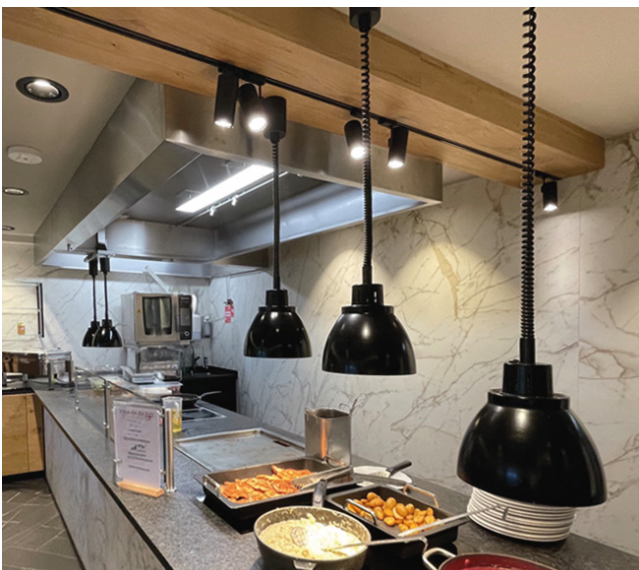
Single kitchen hood in the serving area
